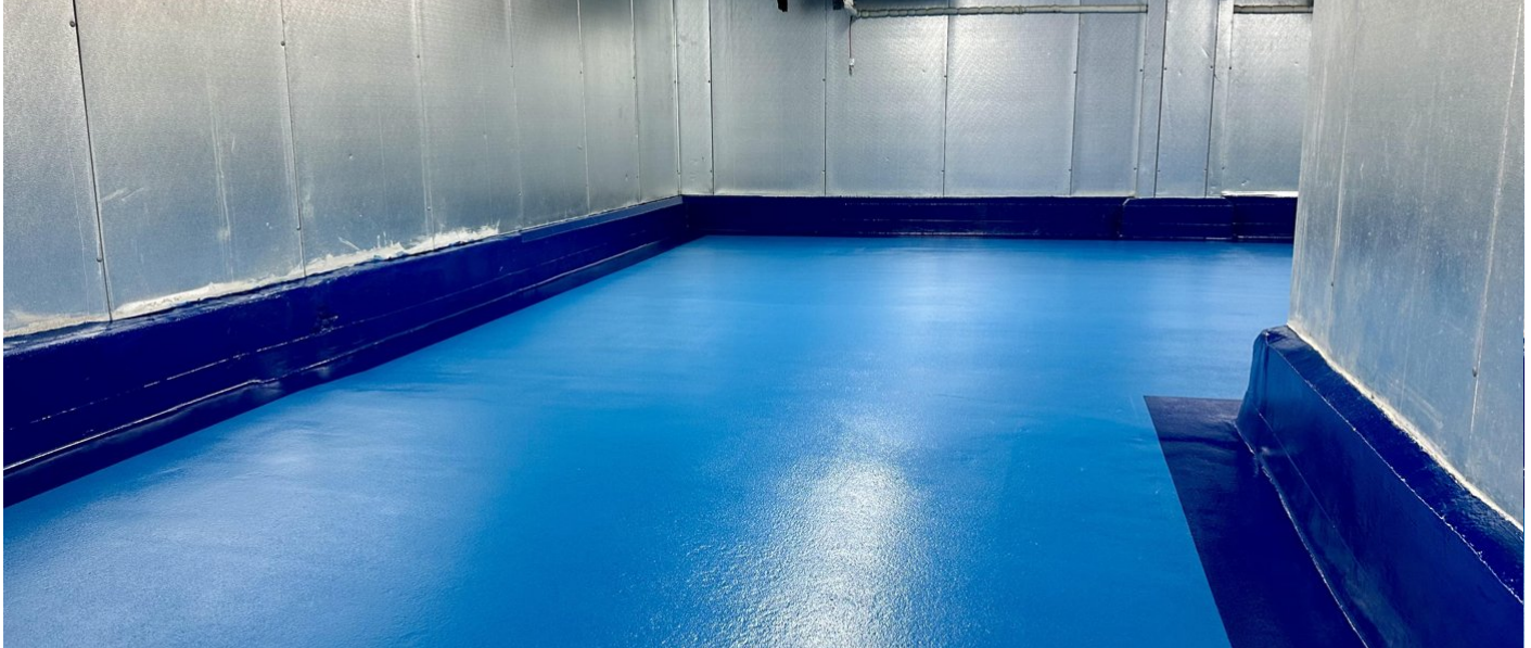
Urethane cement with integral cove base in a cold storage walk-in.
